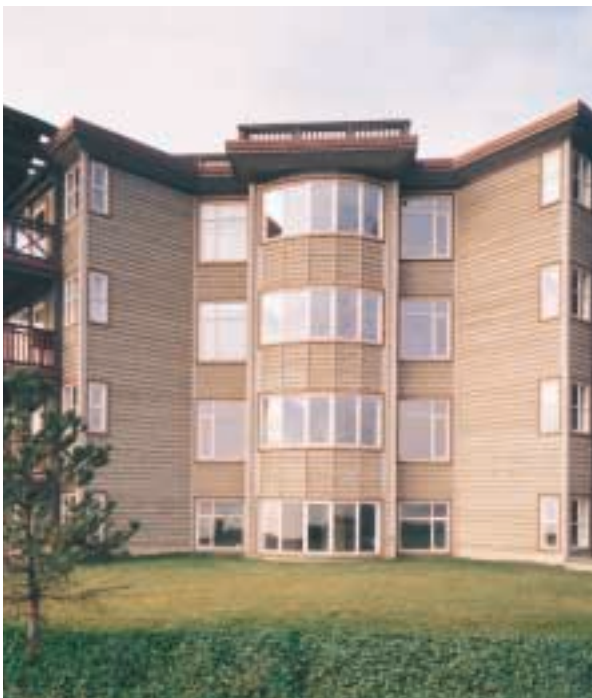
Bevel siding on a large, four story apartment complex. Oil based stain finish.
